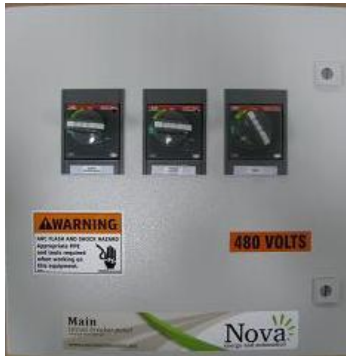
Figure 2 Main Disconnect Panel Front View
