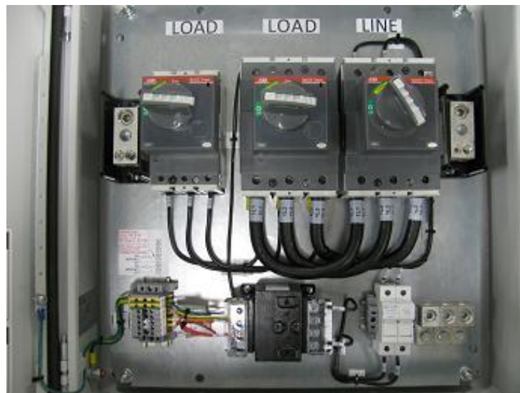
Figure 3 Main Disconnect Panel Interior View
