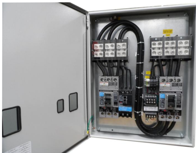
Figure 2 Main Disconnect Panel
