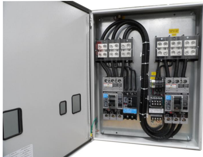
Figure 2 Main Disconnect Panel
