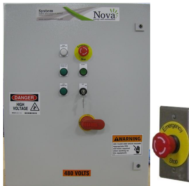
Figure 2 Nova Auto Restart Main Disconnect Panel
