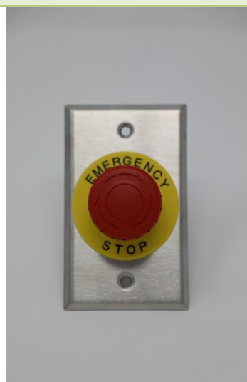
Figure 1 Nova Emergency Power Off Control Station
