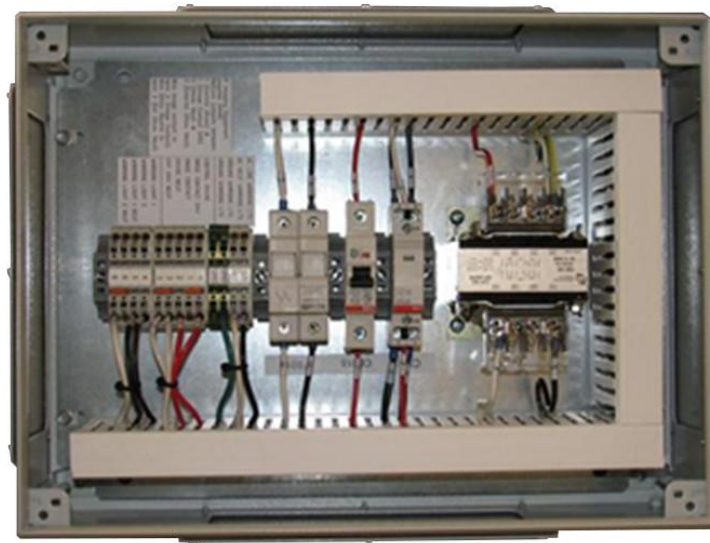
Figure 2 Nova Warning Light Controller- Inside
