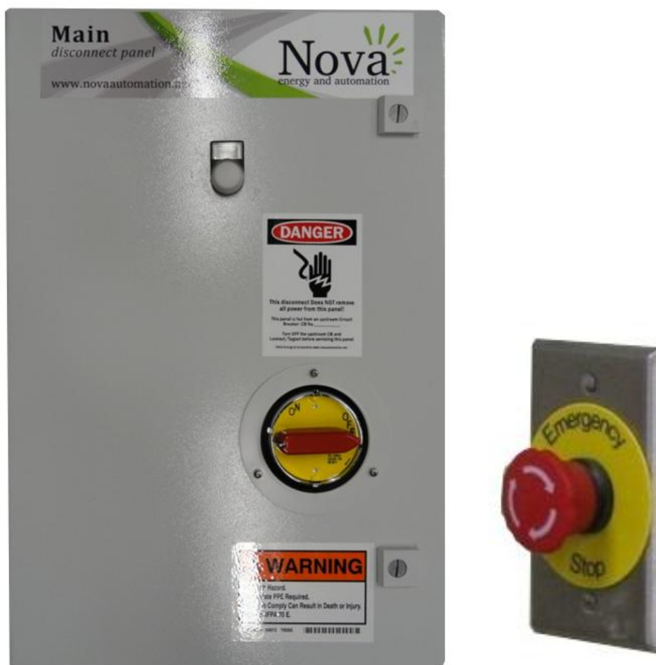
Figure 4 80A Main Disconnect Panel Front View
