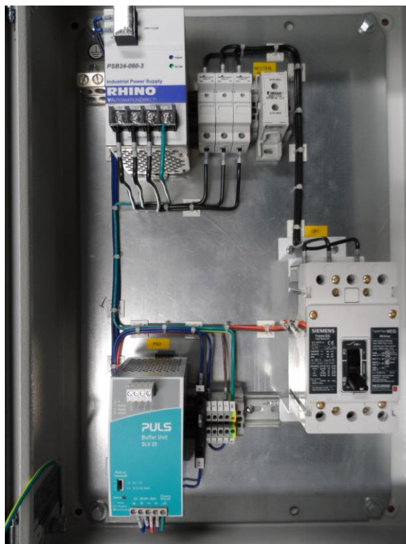
Figure 5 Enclosure Interior Components
