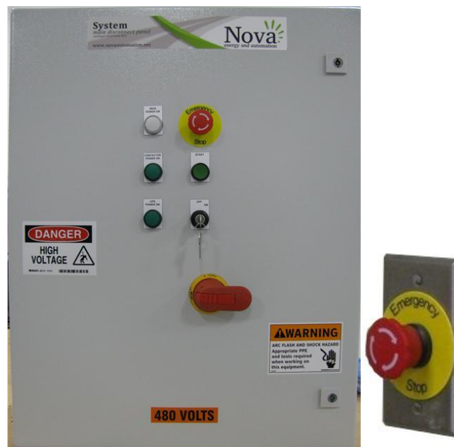
Figure 2 Nova Auto Restart Main Disconnect Panel
