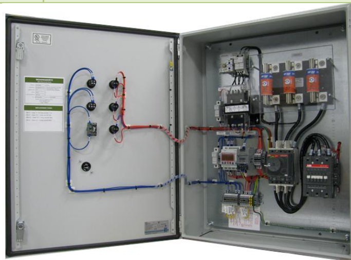
Figure 3 Nova Auto Restart Main Disconnect Panel- Inside
